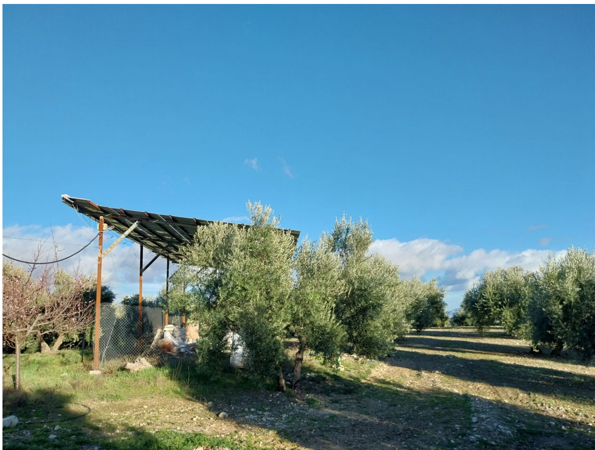
Small-scale solar panel installations among olive trees in rural Andalusia, Campotéjar
